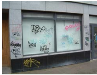
Defaced window and doors
